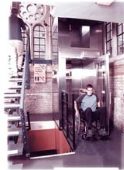
Platform lift installed at Cambridge Corn Exchange
